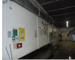
Photo of non-conformity Rain water dripping from shilling.JPG
