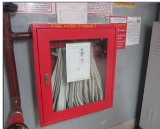
Photo of fire safety equipment Fire hose reel.JPG
