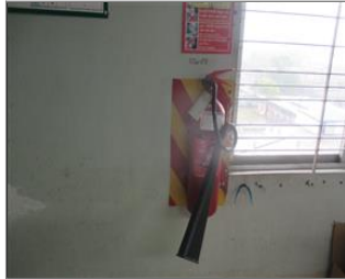
Photo of fire safety equipment Fire extinguisher.JPG
