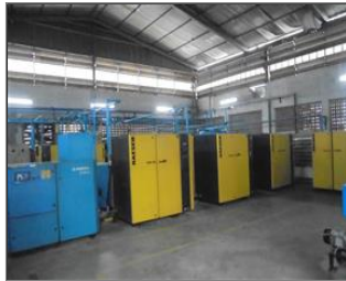
Photo of the inside of the main production hall Compressor room.JPG
