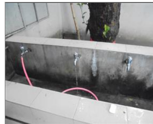
Photo of non-conformity Water falling with no reason.JPG
