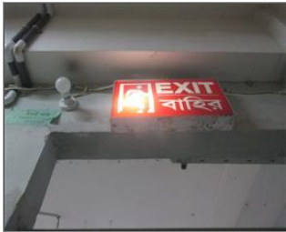
Photo of fire safety equipment EXIT sign.JPG
