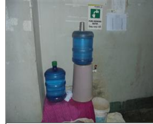
Photo of the sanitary facilities Drinking water.JPG
